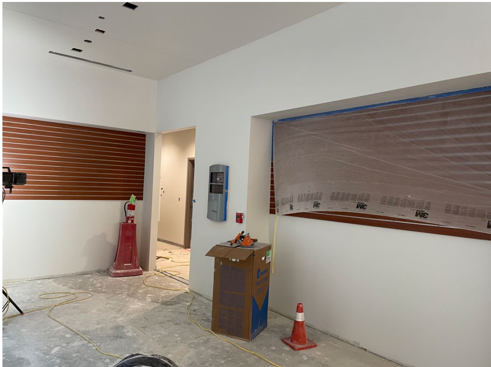
Front Entrance Display wall & "New" Fire Panel
