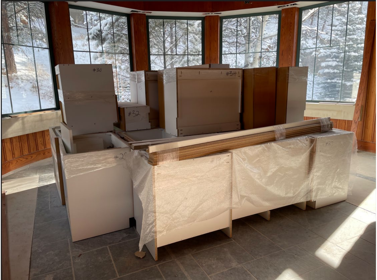
Cabinets on site, ready for install
